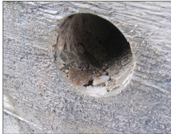
Fig. 4: Detail of the drillhole – patchy concrete.
