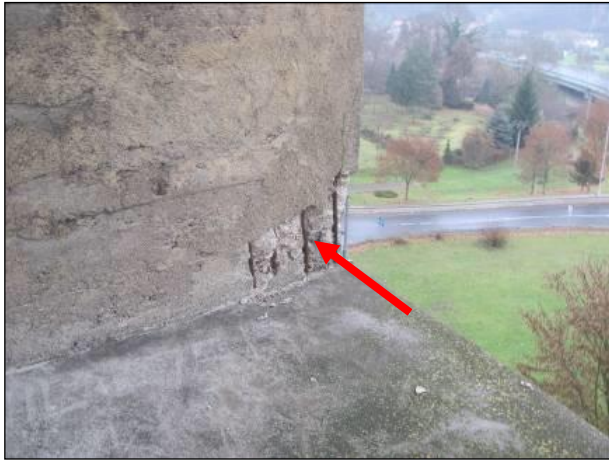
Fig. 3: Deep corrosion of the reinforcement.
